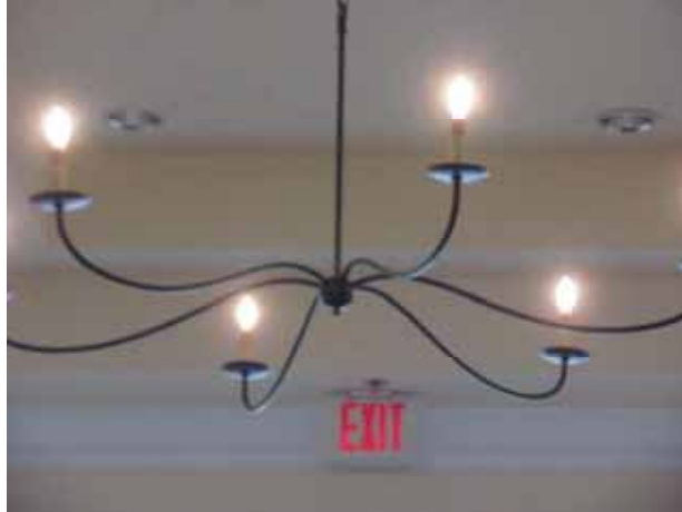
Suspended light fixture
