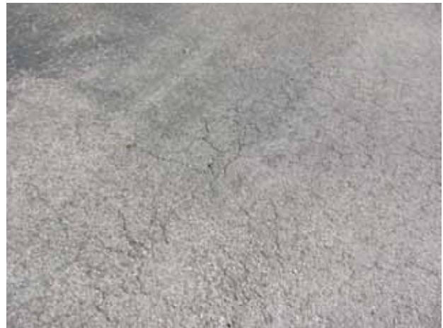
Asphalt pavement at clubhouse – Note cracks
