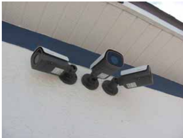
Security system cameras
