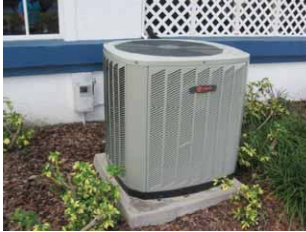
Split system condensing unit
