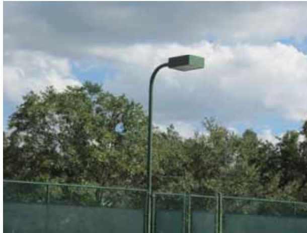
Tennis court light pole and fixture
