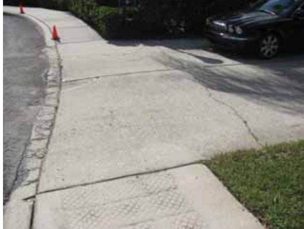
Concrete driveway – Note crack
